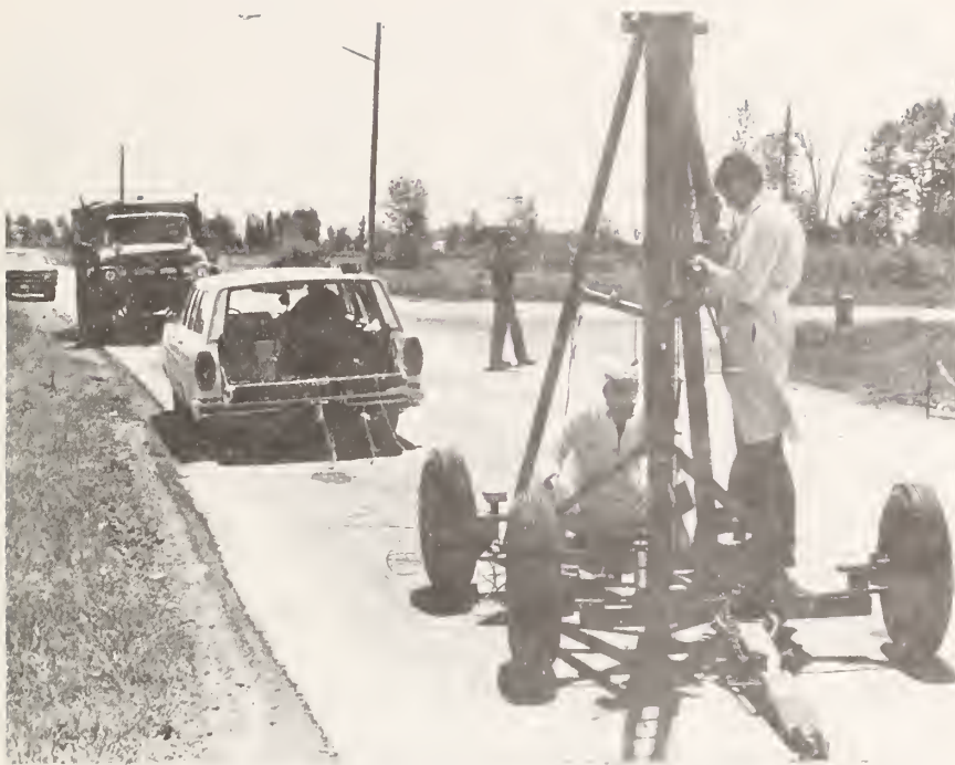
Figure B.24 CAL impulse generator
